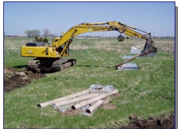
ASBESTOS SEWER PIPES
